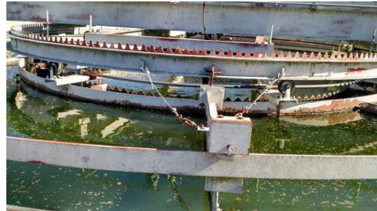
Figure 8b: Shows Clarifier in operation.
