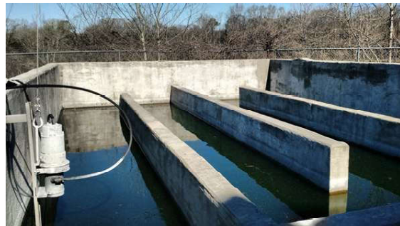
Figure 9: Detention Basin in which chlorine is.
